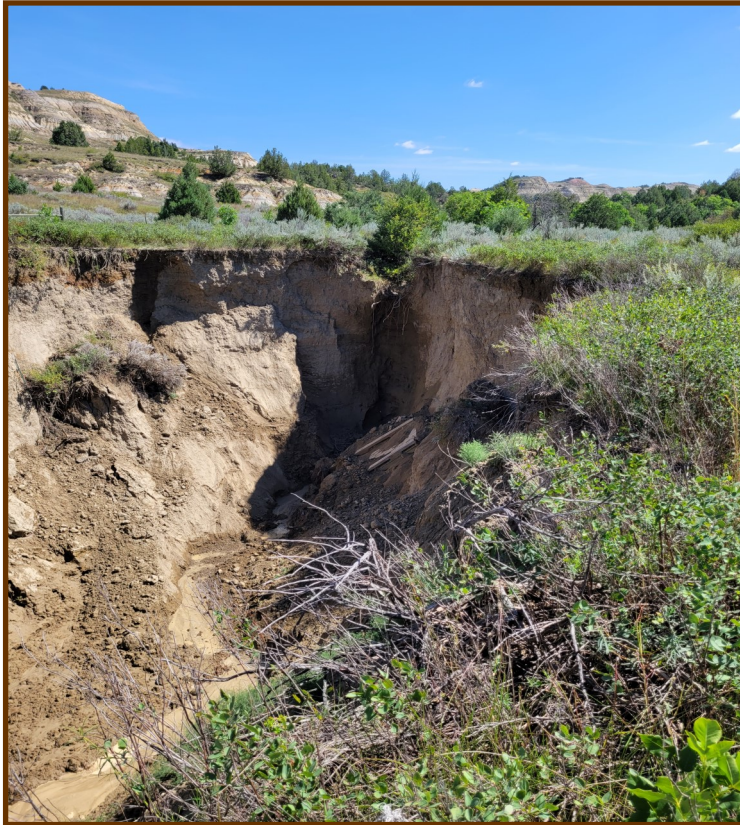
Bridge collapse at 19.5—note bridge at center of picture in the wash out about 50 feet below the trail. Photo taken August 14, 2023 by Pat Ashley
